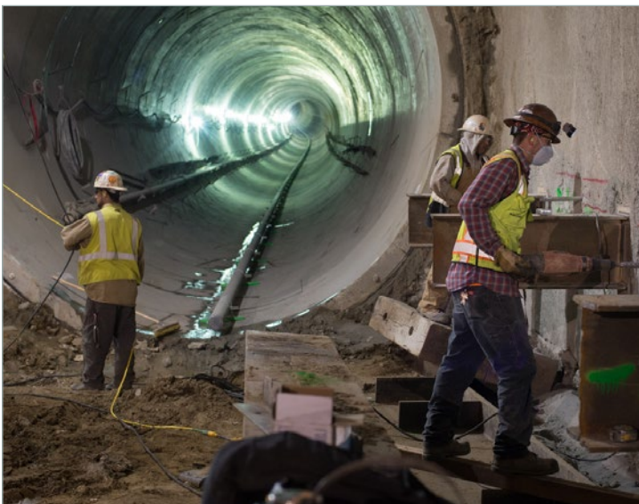
Construction of the Central Subway's Yerba Buena / Moscone Station in San Francisco (Photo: Courtesy of SFMTA)
