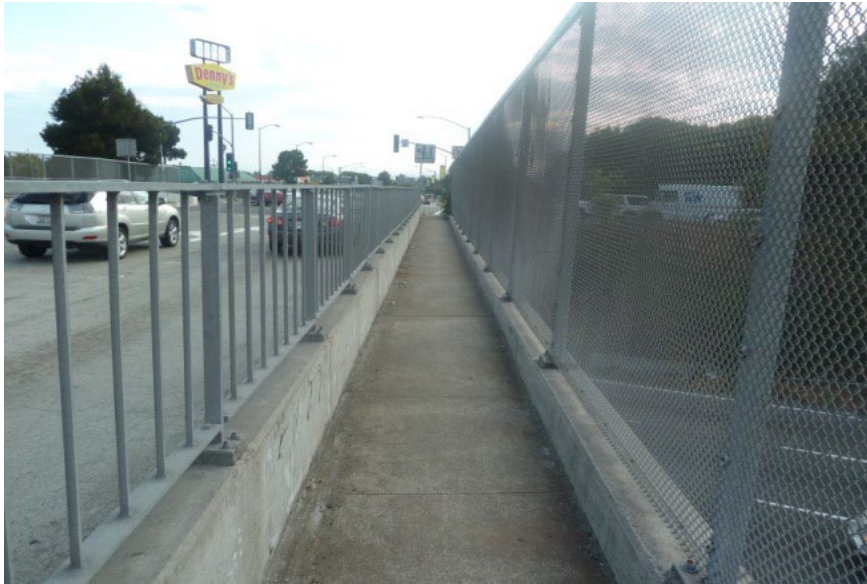
Figure 14. On SPDR overcrossing looking west, with 4-foot-wide sidewalk on north side of structure. Photo credit: AECOM.
