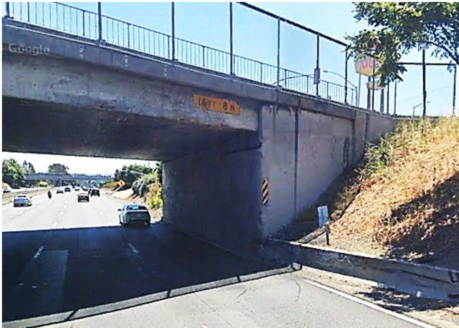
Figure 8. Looking south at SPDR overcrossing from westbound I-80. Scarring of the bridge soffit from truck strikes is visible below the vertical clearance sign.
