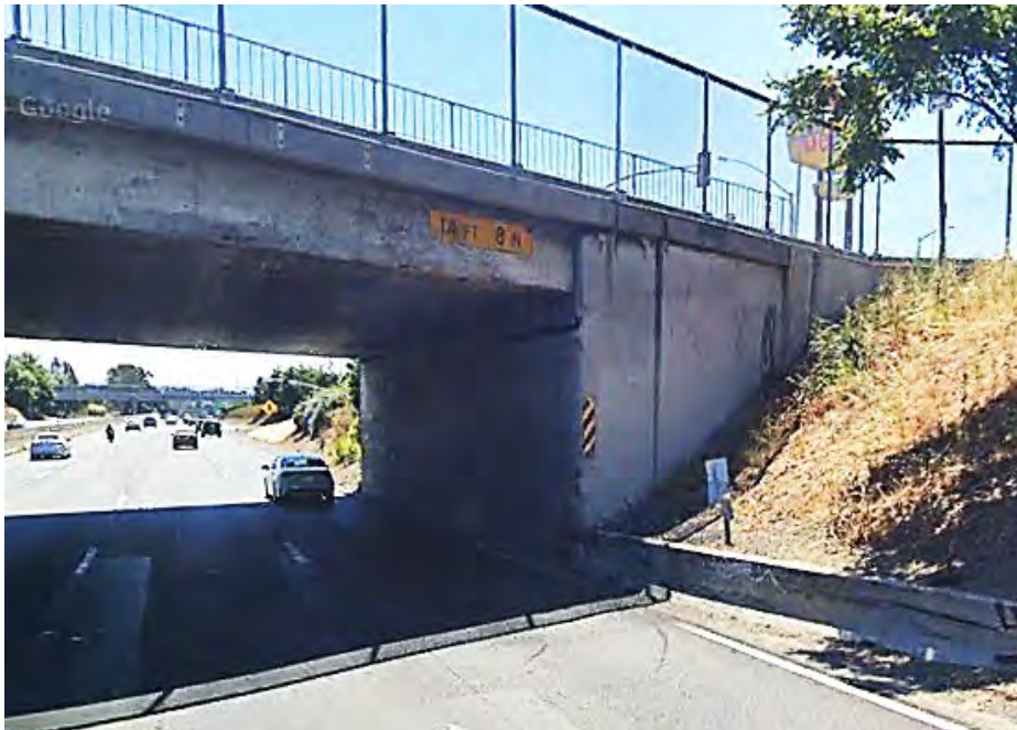
Figure 8. Looking south at SPDR overcrossing from westbound I-80. Scarring of the bridge soffit from truck strikes is visible below the vertical clearance sign.
