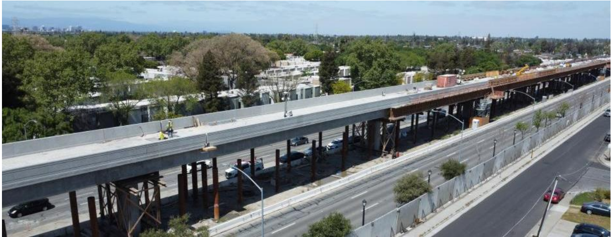
Aerial view of the Eastridge to BART Regional Connector superstructure under construction Photo: VTA
