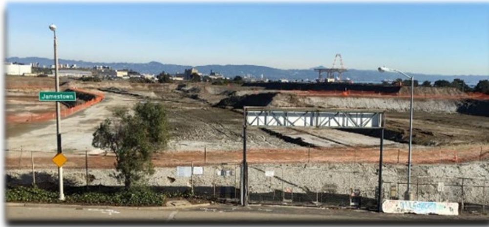
Former site of Candlestick Park Stadium, looking northeast from Jamestown Avenue and Harney Way.
